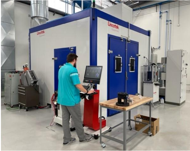
Thermal spray booth
